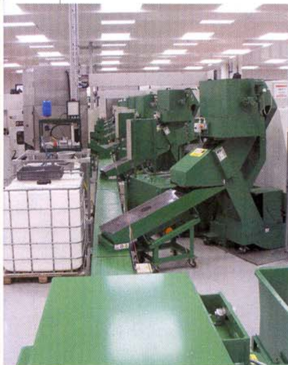
With more space available at Stonehouse, Renishaw has been able to implement a centralised swarf system
